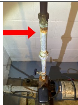
Recommend updating rusted nipples
