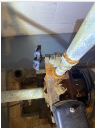
Main water shut off valve
