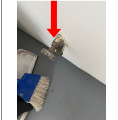
Handle is stuck on the hose Spicket in the garage
