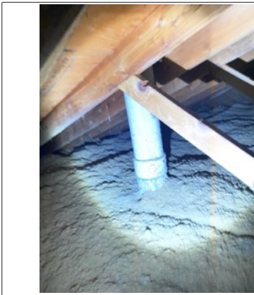
Asbestos beltline. Recommend not disturbing
