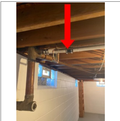
Negative slope in the drain line
