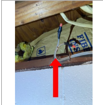
Recommend removing wire that is no longer used. Double tapped into pre-existing breaker
