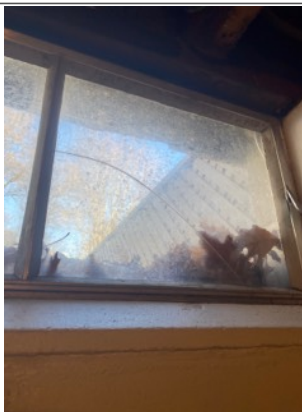
Cracked basement window
