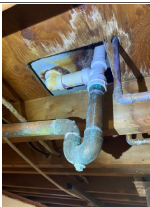
Recommend monitoring or updating Rusted plumbing underneath the bathroom
