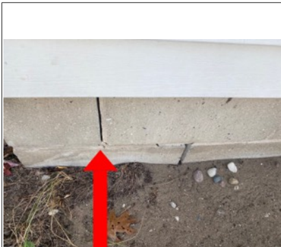
Recommend Tuckpointing missing mortar joints
